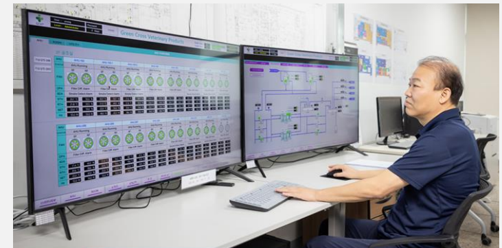
R-320, BMS room
