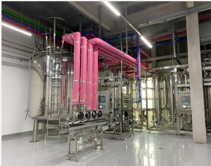
R-305 Water treatment room
