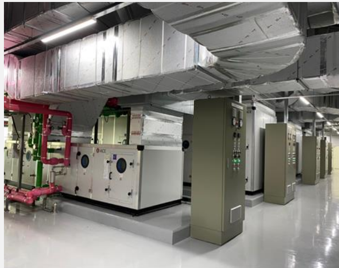
R-304 HVAC room II
